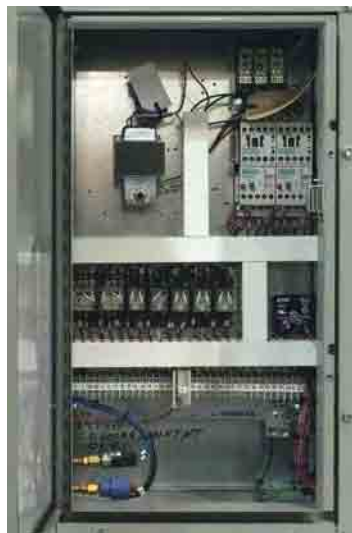
Organized electrical cabinet provides easy service and maintenance.
